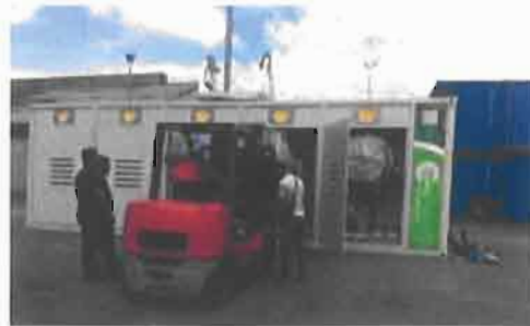
Microturbine equipment to be installed upon completion of civil works
